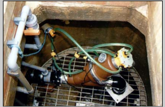
Iseki Redivac Interface Valve installed in chamber
