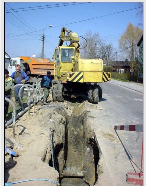
Installation underway in narrow trenches Cost effective solutions to many difficult drainage problems.
