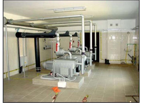
630 m 3 /hr vacuum pumps
